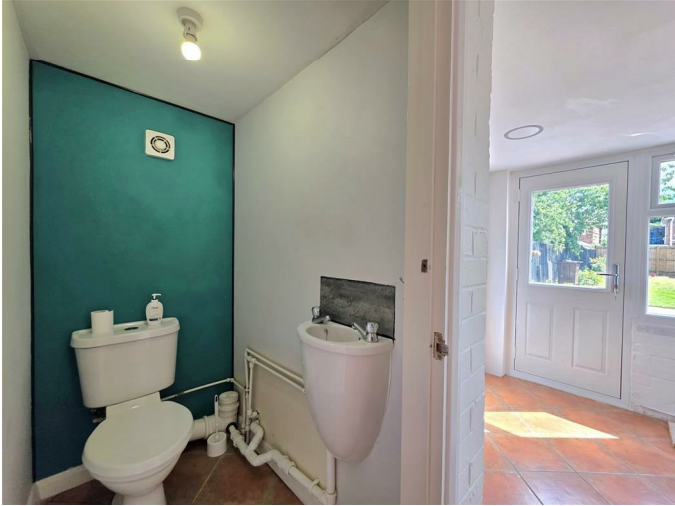
Tiled flooring. Toilet. Wash hand basin. Extractor fan.
