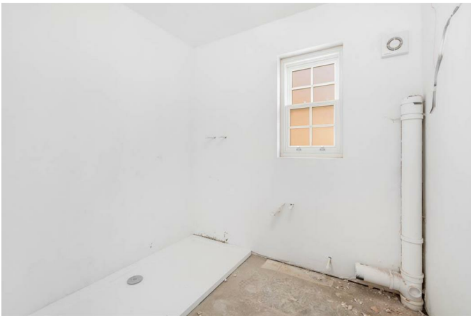
Shower cubicle. Wash hand basin. Toilet. Heated towel rail.
