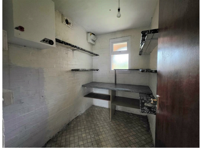
PVC double glazed window to front, wall mounted electric consumer unit, wall mounted oil central heating boiler.
